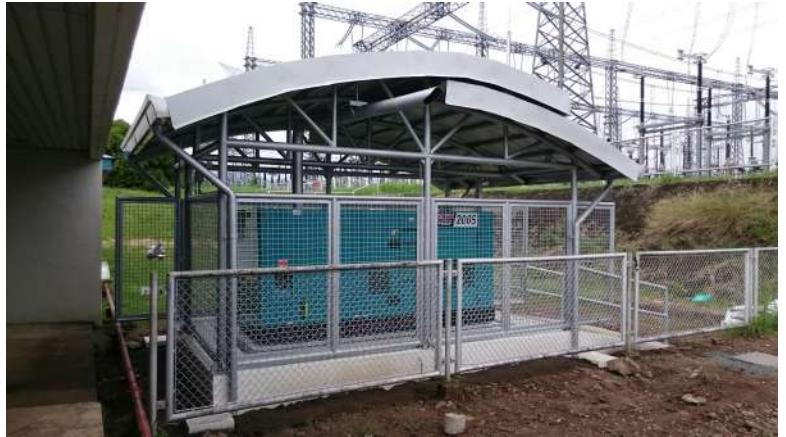
A Powercity 200 KVA generator and air-cooled steel shelter supply project of Powercity Corporation in a power grid.
