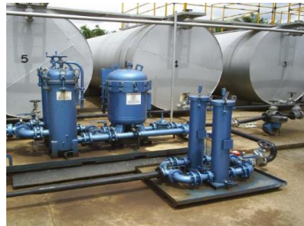
An example of large capacity, complex and permanent FP system.
