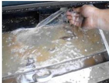
Figure 4. Water drained from a generator tank.
