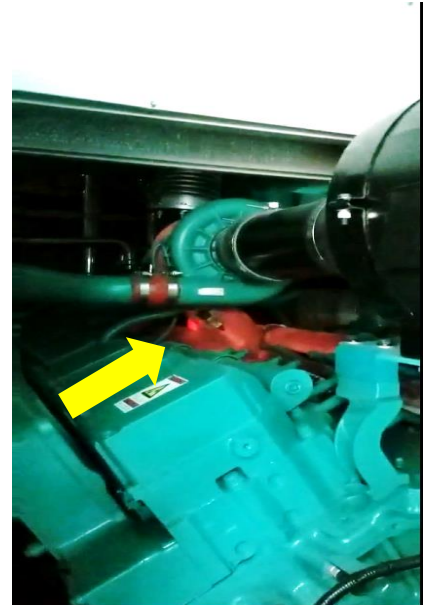
An overloaded generator set with smoldering turbo and exhaust manifold.
